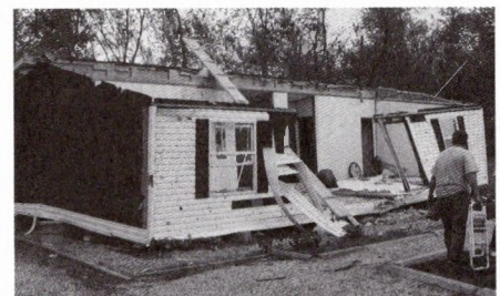
The team helped demo this house in Fairfield. A car had landed in the living room.
